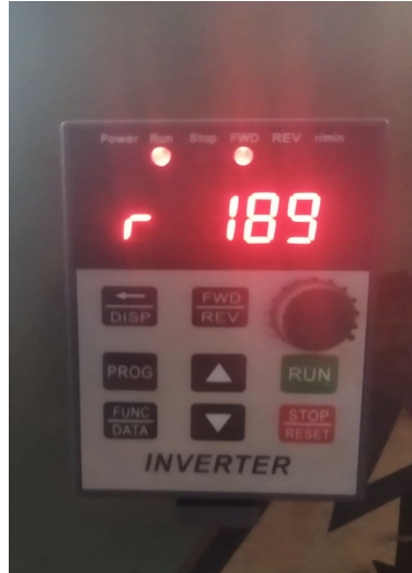
Gambar 7. Panel Kontrol VFD Posisi RUN
